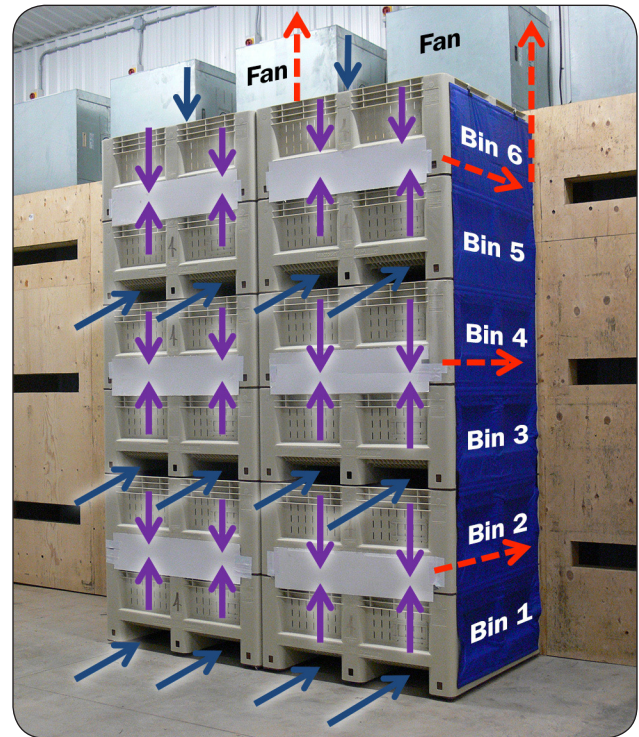
Figure 4. This serpentine horizontal/vertical airflow system has centrifugal fans inside metal housings above a plywood plenum. These fans pull refrigerated air through “hot” tree fruit in plastic bins. Each stack of six bins is independent. Three forklift openings across from wall slots are closed off with coverings. This compels cold air to enter through the remaining three open forklift openings and travel up or down through the fruit via slots in the bin floor. As the air warms (purple arrows), it is directed back into the storage room (red arrows) towards the evaporator coils to be re-cooled. Bins are tightly stacked so no air can short-circuit through the bins’ side vents. If stacks are missing, a tarp is installed to prevent short-circuiting. This tarp can be seen covering the sides of the right column of bins. The system shown here is under construction, as foam padding around the slots is to be installed. (Photo by Hugh Fraser, OMAFRA)
